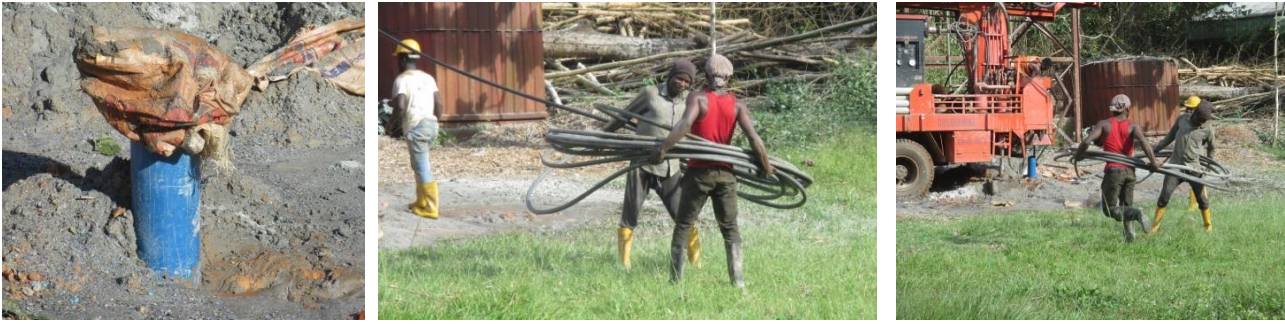
Borehole Completed; The borehole pipe was temporarily covered once drilling was done, as the process was not yet finished for Engineer Chris. However, once the drilling was done, the borehole workers cleaned up by having a little fun rolling up the drilling material.
