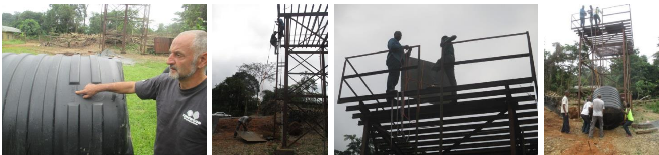
Water Storage Tanks; Two 3000 liter water tanks were placed on the tower - but first steel plates were laid down to stabilize the tanks.
