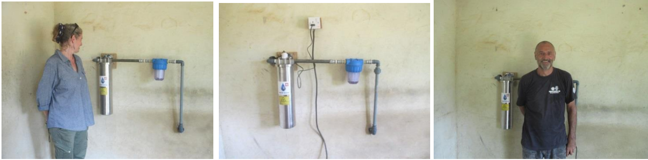
The Water System; The centerpiece of the system, the Aqua Pura Waterflow system is now installed and connected. Information on this fantastic water purification plant can be found at www.aqua-pura.org . Our project was featured in their April 2016 and December 2016 blogs at https://saubereswasser.wordpress.com .
