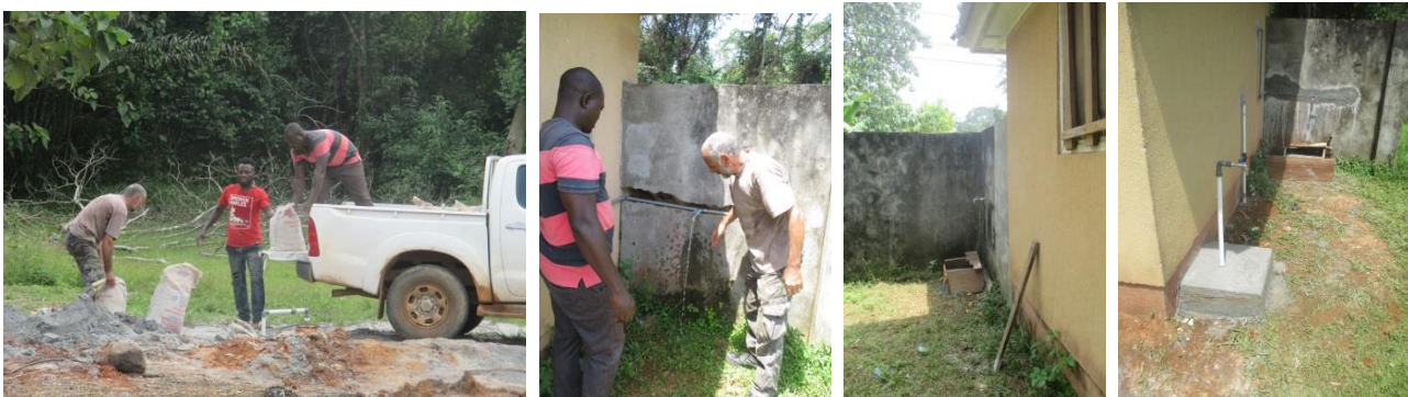
Platforms for Placing Basins; Finally, cement platforms for the water canisters were placed. Rangers and the community can now obtain clean, bacteria-free water, free of charge.
