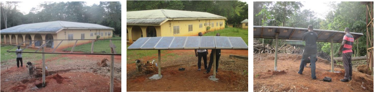
Solar Panels Mounted; The mount for solar panels was created by a local welder and the solar panels assembled and connected by the engineer of this project, Chris Jukpah.
