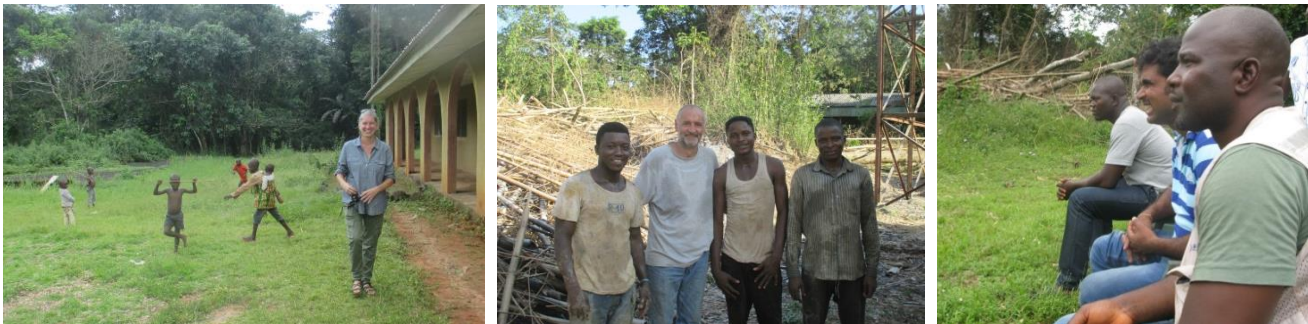
The Drilling Crew; The drilling process was documented by Dr. Kathy Wood with the help of some of the local children. The hard-working drilling crew is pictured with Bruno Tenger in center. On right, Engineer Chris Jukpah, with the drilling crew, kept a close eye on every step of the work.
