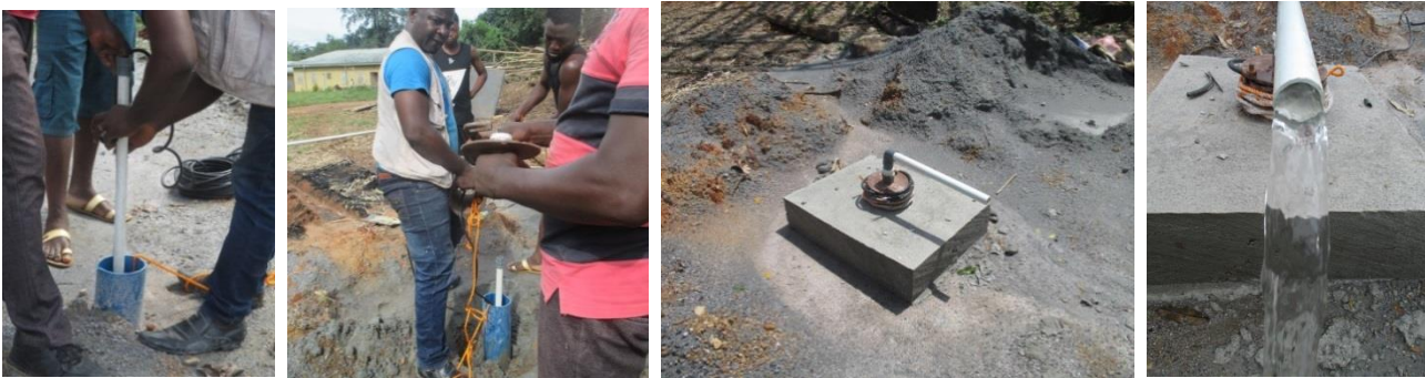
We Have Water! The solar pump was then immersed deep in the borehole, followed by cementing and sealing. Our first test of the system with a generator and water flows! A very good moment!
